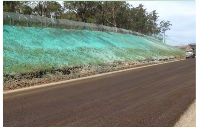
Ameliorated Application being applied to the Hunter Expressway (Kurri Kurri to Branxton project)
