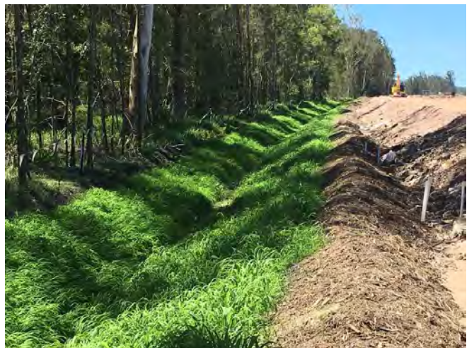
Figure 16 - Fill 13 NB Drain 10th Nov 2015 after 173.3 mm Rainfall since 29th Sept 2015 - Dense healthy grass on loose topsoil surface
