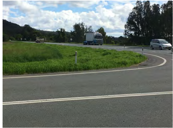
Figure 7 - Pub Intersection - 10th Nov 2015, Dense healthy grass on loose topsoil surface.
