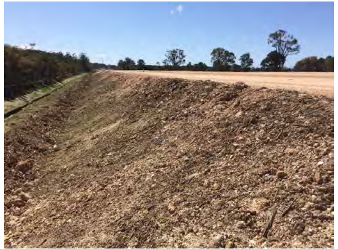
Figure 12 - Fill 13 NB 29th Sept 2015 after 97.2 mm Rainfall since 16th Sept 2015 - Germination evident on face, more pronounced on topsoil areas.
