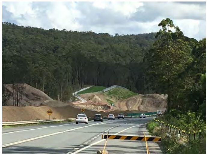
Figure 4 - Cut 19 NB Ameliorated Mix Application, Upper Batter 10th Oct 2015, Lower Batter 29th Oct 2015
