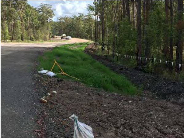
Figure 6 - Blackmans Point Rd Interchange SB - 10th Nov 2015, Dense healthy grass on loose topsoil surface
