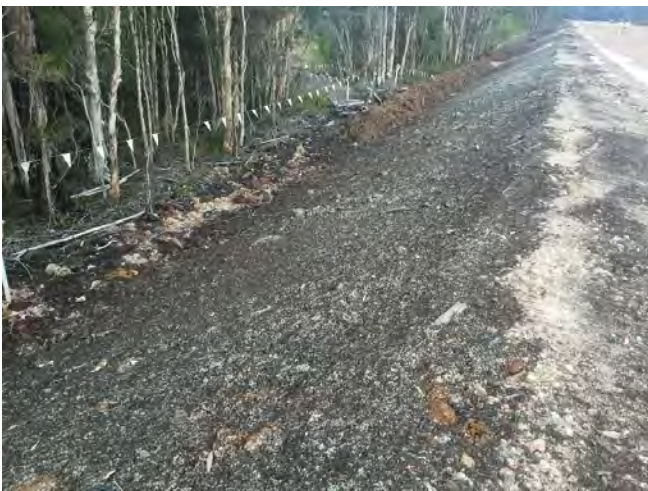
Figure 11 - Fill 13 NB 16th Sept 2015 after Initial Rainfall - Application no longer visible on surface, allegedly washed down batter into wood chip berm
