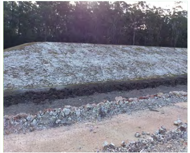
Figure 2 - Cut 5 NB Nov 2015, Failed Standard Specification Mix
